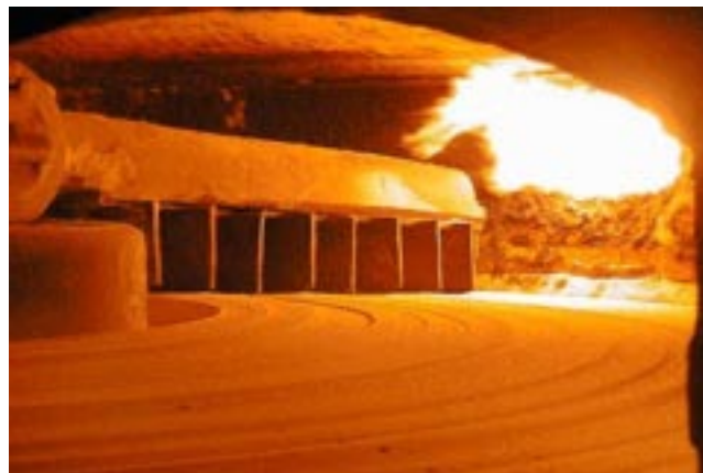
An inside look at one of three MOLYMET's roasting furnaces in a production complex located south of Santiago, Chile. (Photo Courtesy of MOLYMET, Chile.)
