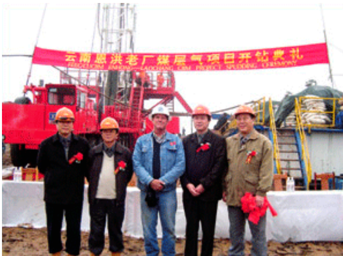
FEEC and Chinese officials mark the start of drilling on site in the Yunnan Province of Southern China
