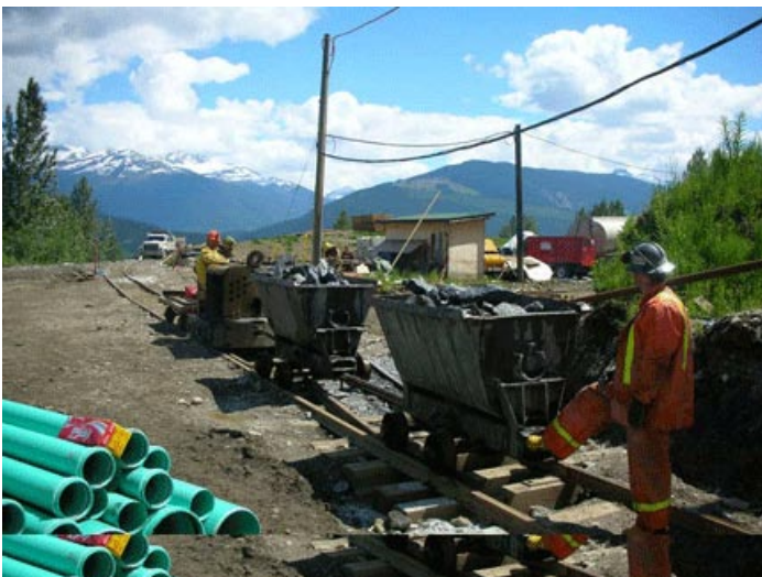
Roca Mines plans to be Canada's newest primary molybdenum producer in the fall of 2006 at Trout Lake in British Columbia
